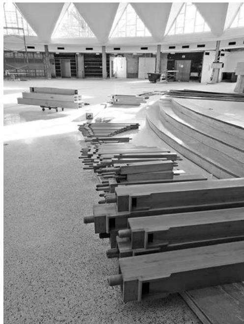
Sets of organ pipes from the Cathedral of St. Joseph's previous, 1968-vintage pipe organ are placed in the middle of the Cathedral, which is undergoing a major renovation, in this photo from Feb. 1. These pipes will be reconditioned and incorporated into the new instrument that is being designed and built for the Cathedral. — Photo by Father Jeremy Secrist
